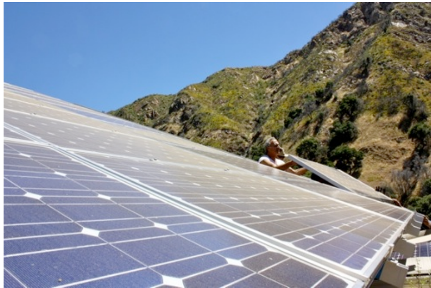
Solar system being installed at Tassajara Zen Mountain Center: Credit Simon Moyes
