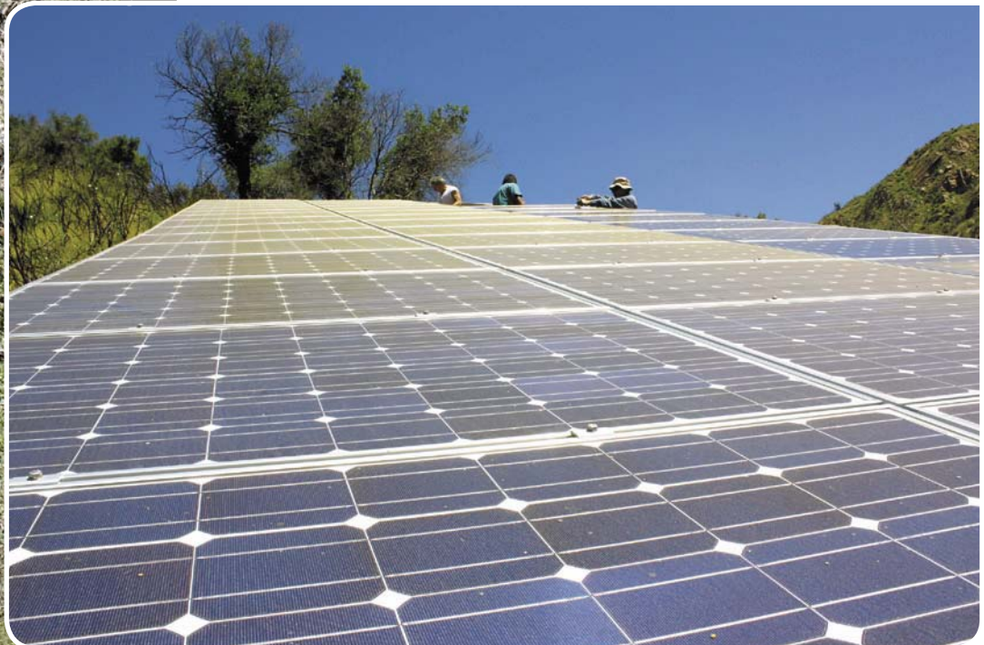
Looking upwards: The 21 kW solar system at the Tassajara Zen Mountain Center is located 90 m above the compound's buildings.
