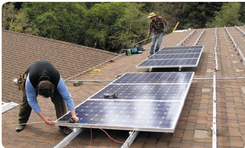
The Lord's work: Workers install part of the 17 kW PV system at the St. John's Episcopal Church in Oakland, California.
